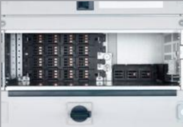
Plug-in busbar system at the compartment rear
