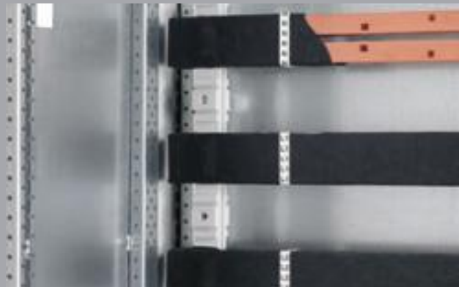
Isolated main busbars
