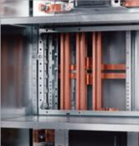
Vertical distribution busbars
